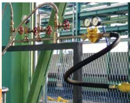
N 2 Purge System
