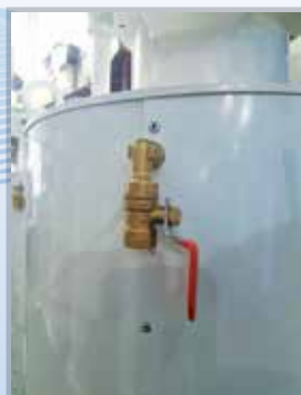
Water Overflow Valve (Prevent the Water Evaporation)
