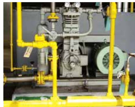
Ammonia Unloading Compressor
