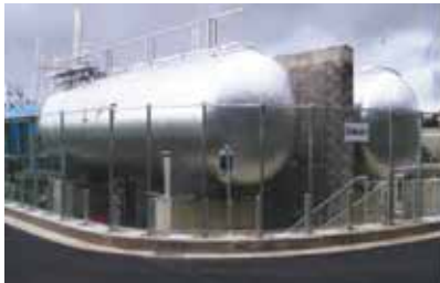
LPG storage facilities
