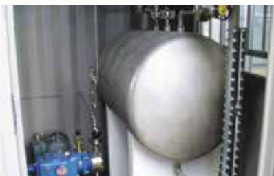
Odorant injection equipment
