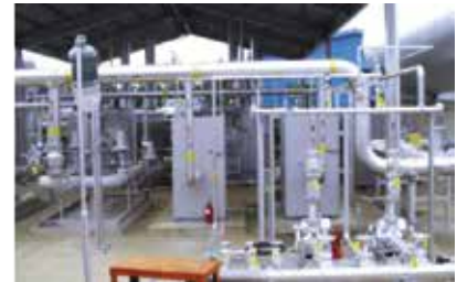
LPG vaporization and mixed equipment
