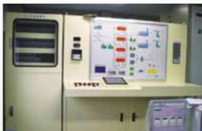
Main control room
