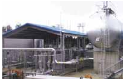
Mixed gas supply equipment
